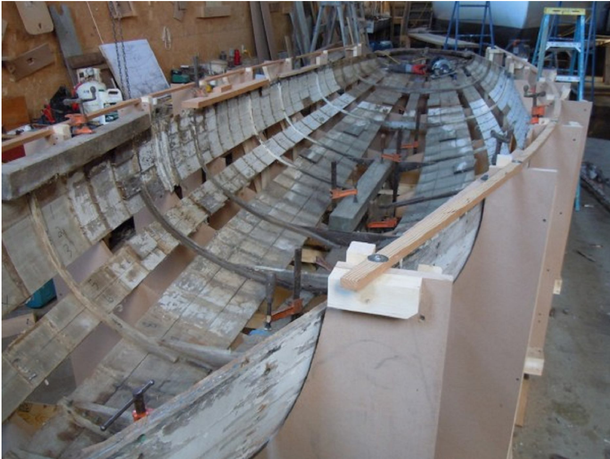
The loosened-up hull was forced out against the molds and screwed there.
