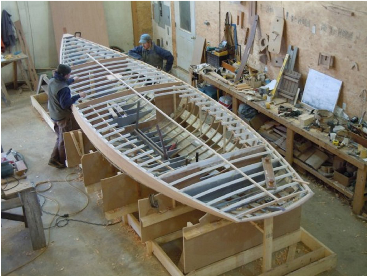
Deck frame is now in, and the deck is about to be laid. Molds were cut down enough to allow hanging the three edge-glued strakes of topside planking.
