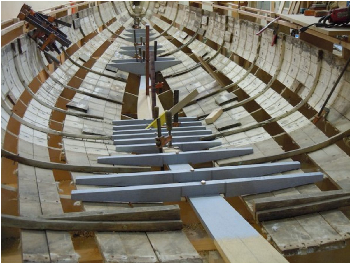
Floor timbers, with shapes taken from the original offsets, go in next—on top of the new keel and temporarily attached to the hull planking.
